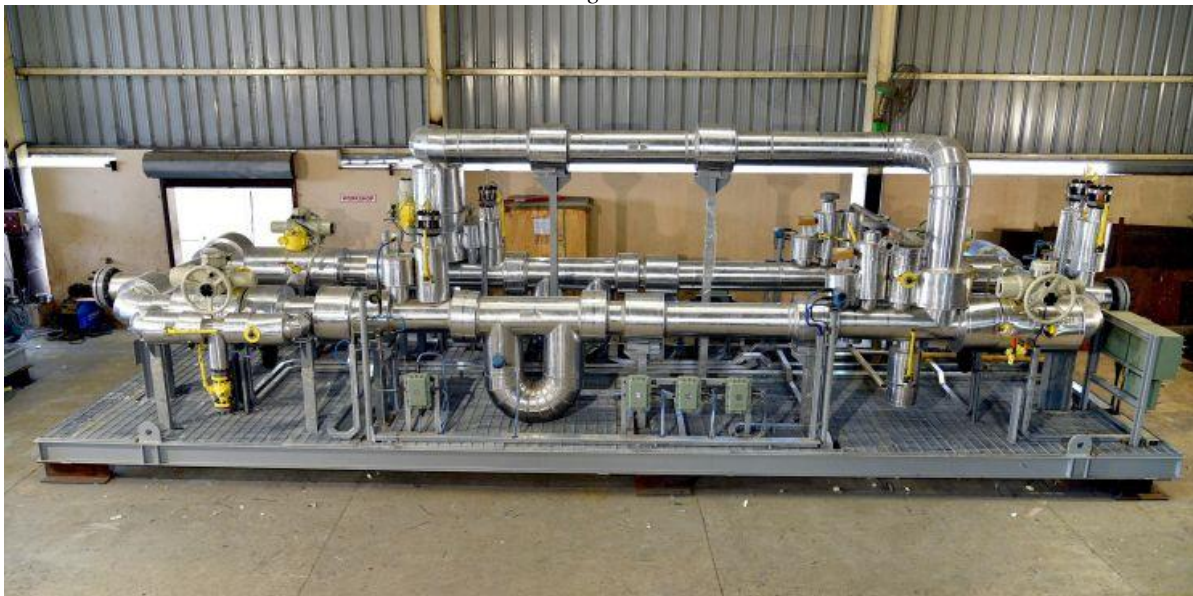
Fiscal metering system
