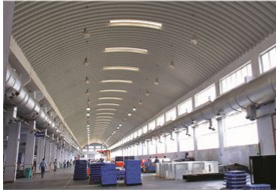
Roof with Hanging Ducts
