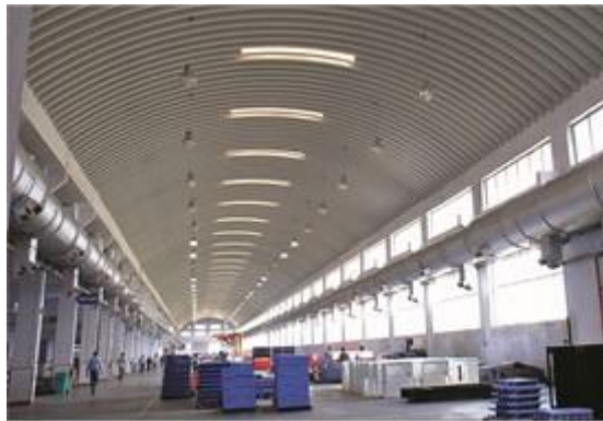
Roof with Hanging Ducts
