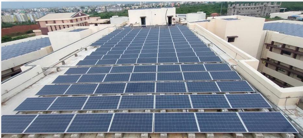
1.2 MW Rooftop Solar Plant at Bhubaneswar, Odisha
